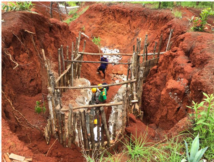
Gully Erosion Control
